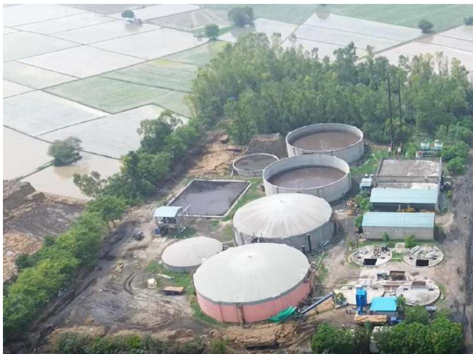
Bio-Gas Generation Plant
